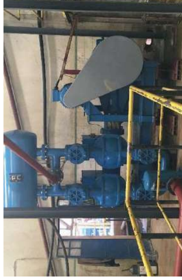
ABEL HM for the Discharge of Tailings Thickeners
